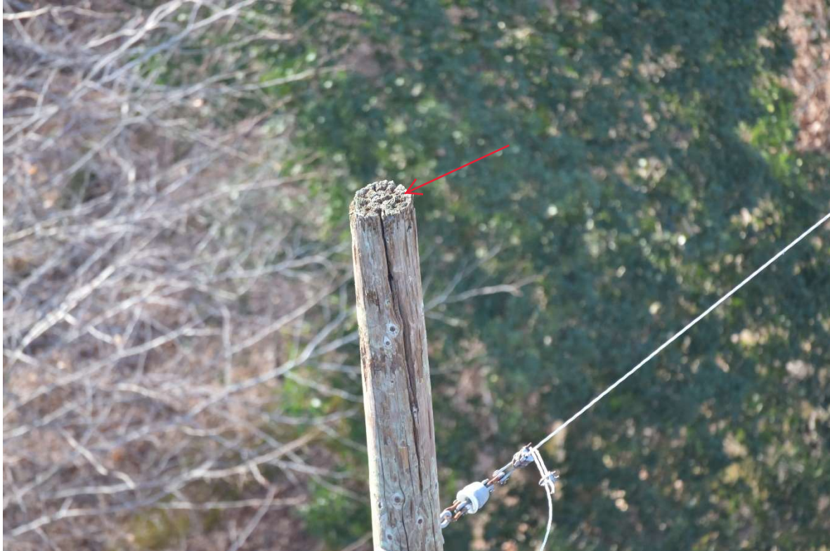
Str 224/24, Rotted Pole
