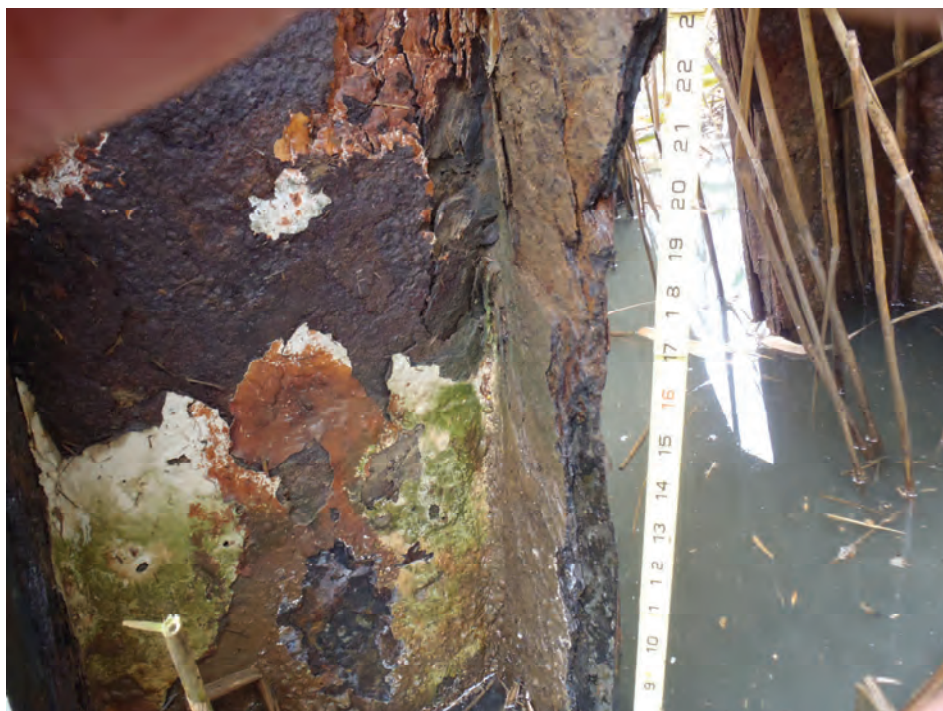
FOUNDATION 4-PILE SECTION LOSS
