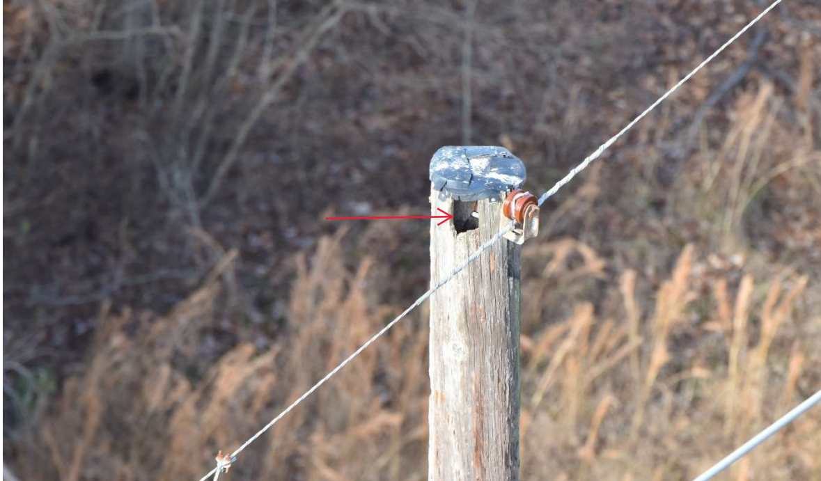
Str 224/287, Rotted Pole
