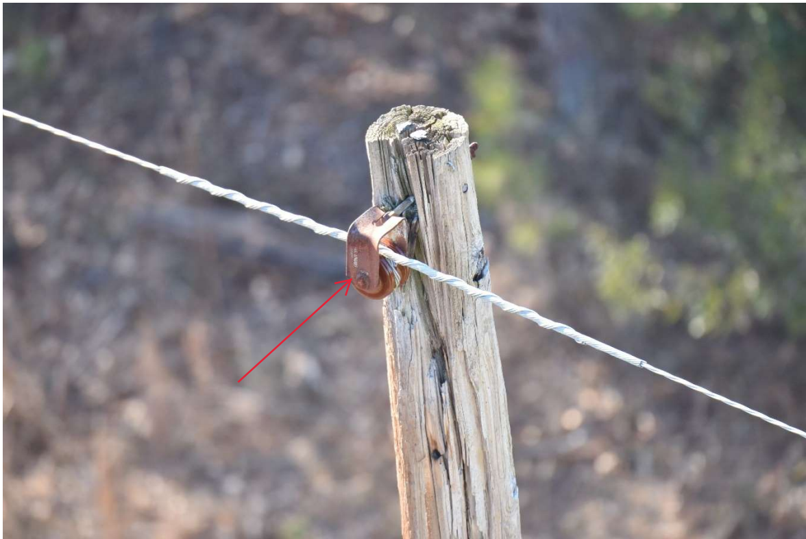
Str 224/122, Weathered static attachment
