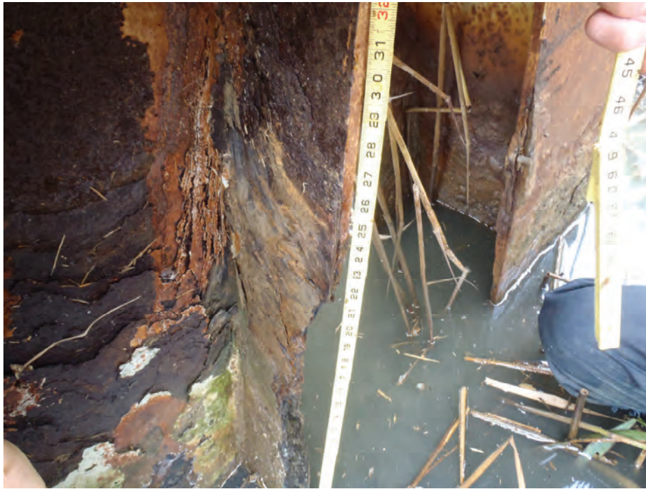
FOUNDATION 4-PILE SECTION LOSS
