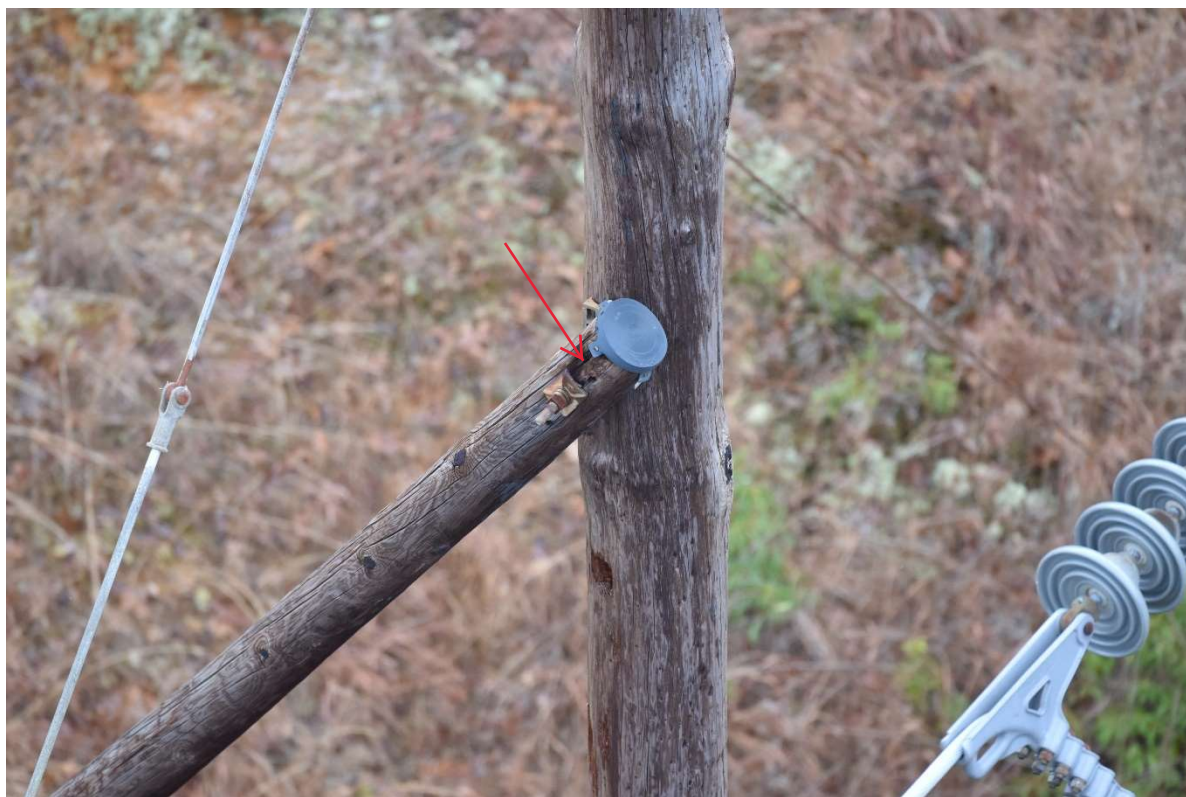
Str 224/81, Rotted cross-brace
