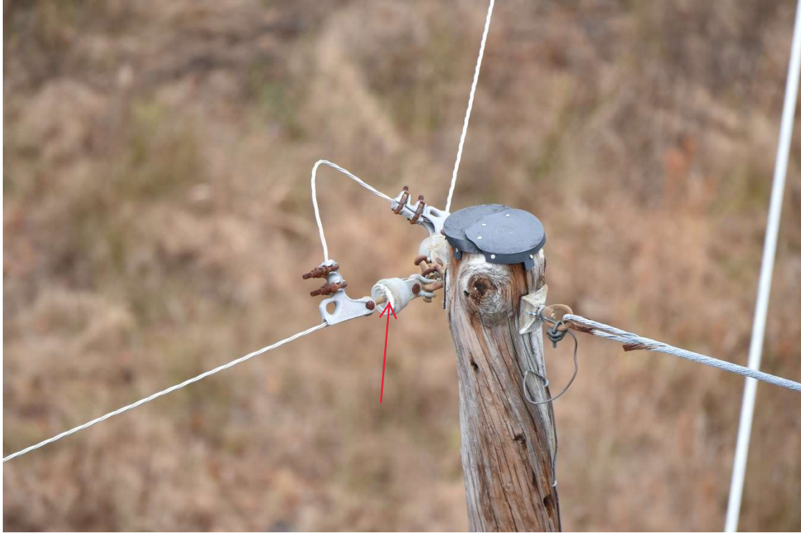
Str 224/66, Broken Static Insulator
