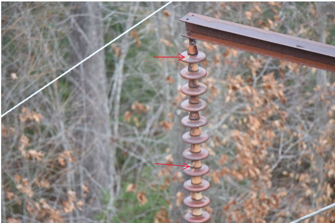
Str 224/80, Flashed Insulator
